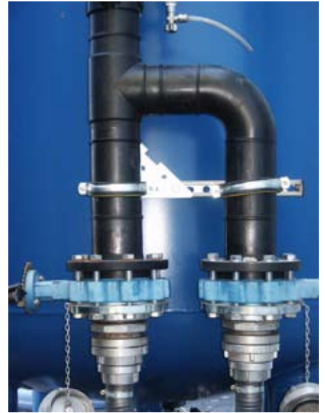
Inlet pipes to the water phase carbon vessel
