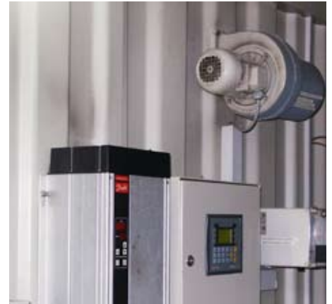
Control panel of the plant (gsm, remote control, data recording) including a second LEL-system at the inlet of the catalytic oxidiser
